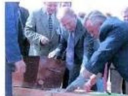
The President of Ukraine L. Kuchma and Governor of Volyn S. Klimentchuk laying the foundation stone in the Perinatal Center basement.
